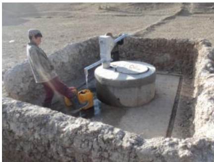
Fig 13 – A completed well – one of the few with a fence constructed around the water point
