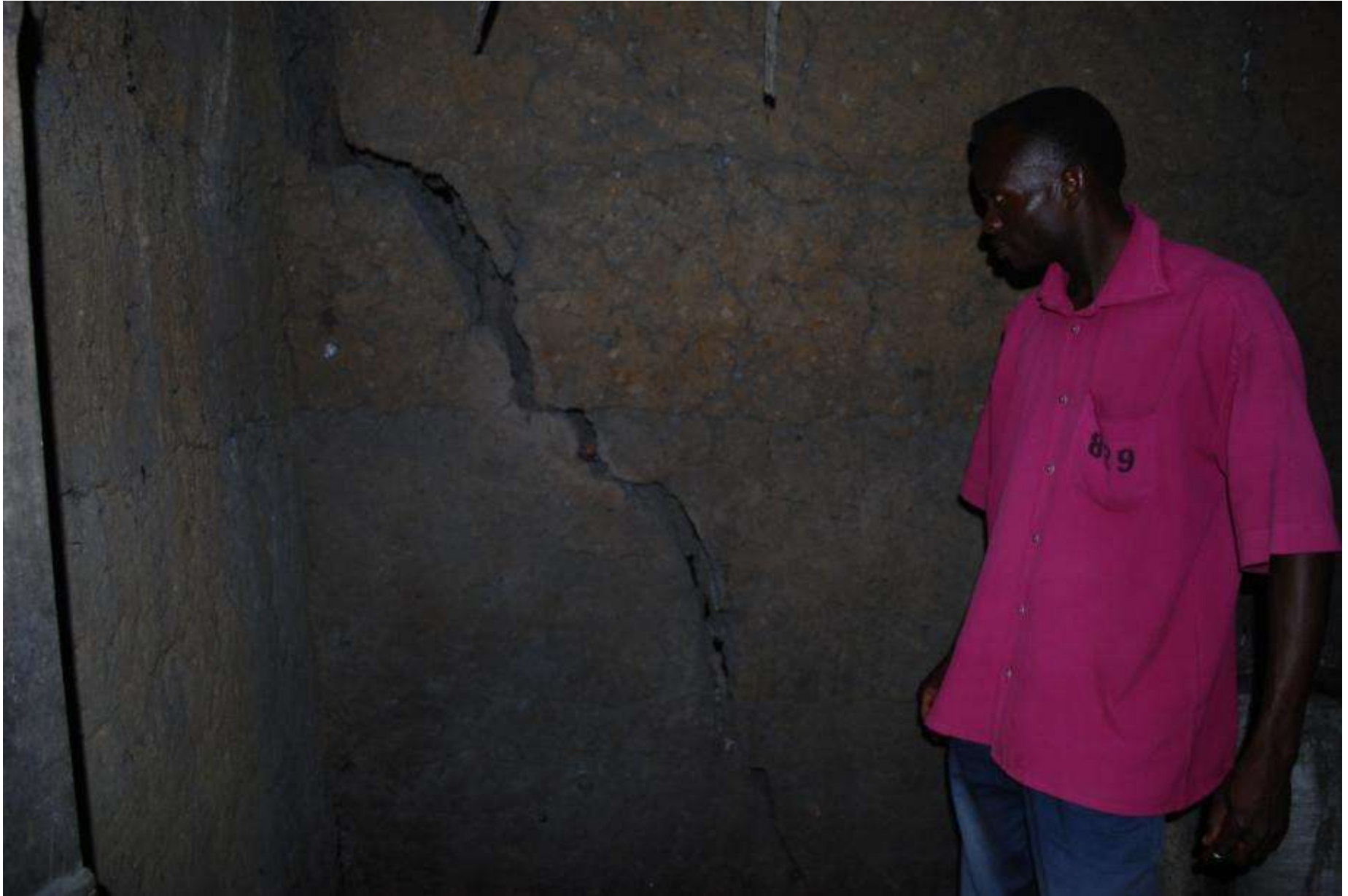
Damage to a house after the 2010 flood
